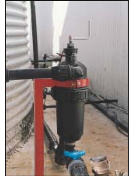
Recirculating of water at a green house.
