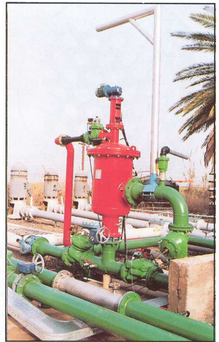
Prefiltration of drinking water treatment. ISRAEL.
