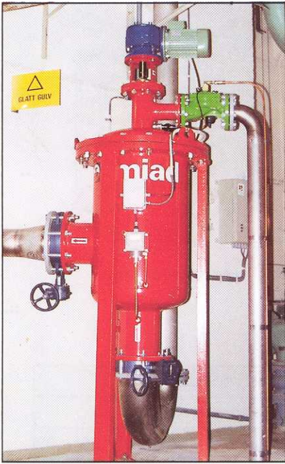
Cooling water in Hydro-electric power station. NORWAY.
