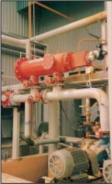
Cooling water in plastic industry, MALAYSIA
