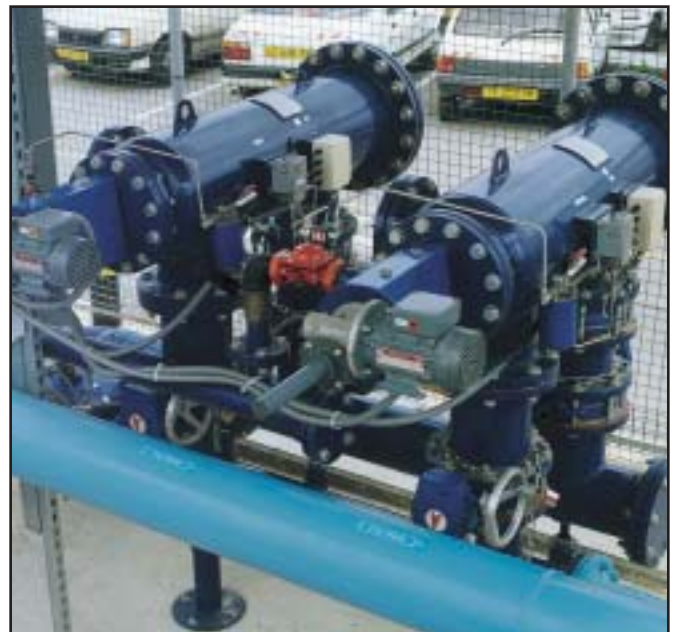
Supply water for semi-conductors plant, ISRAEL
