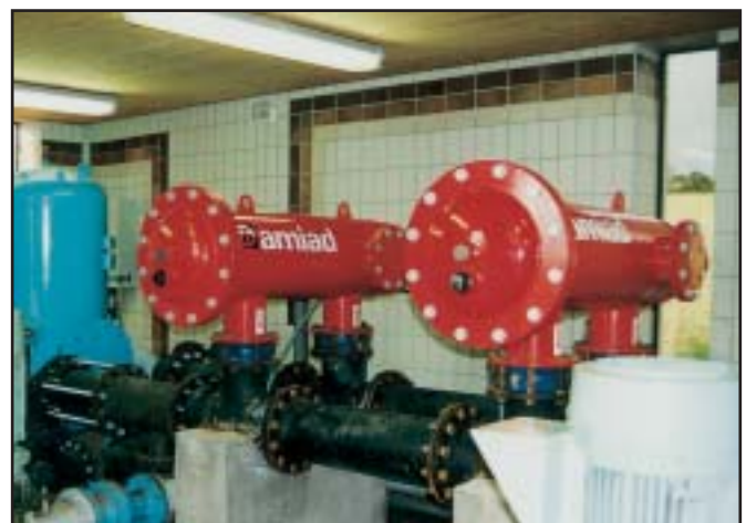
Municipal drinking water, Swinford County, IRELAND
