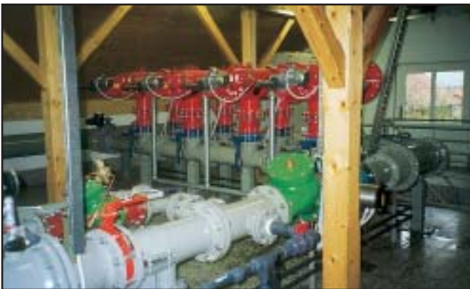
Pre-filtration for drinking water, 10 micron. SLOVENIA
