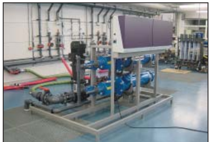
Pre-filtration for UV disinfection, industrial green house, HOLLAND
