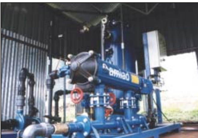
Pre-filtration for water treatment, tea plantation, KENYA
