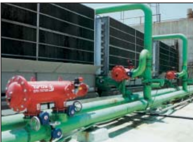
Cooling water for the Central Post Office, ISRAEL
