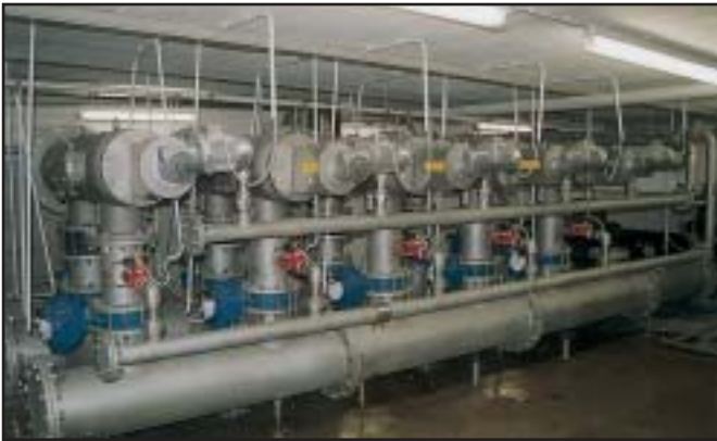
Municipal drinking water, Hallertau, GERMANY
