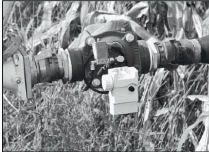
Automated irrigation of a corn field with Cyclik control system.
