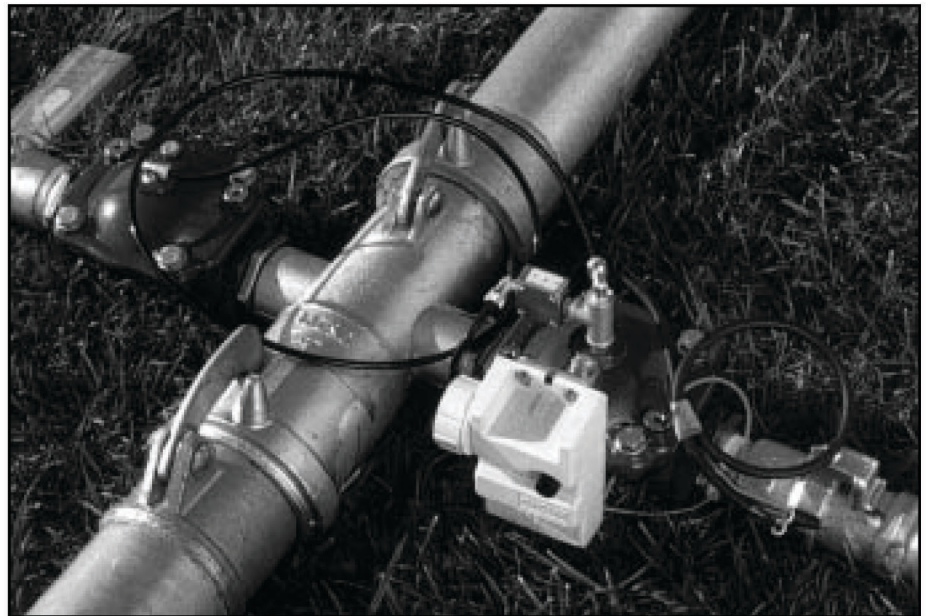
CYCLIK control module shown operating two Rain Bird cast iron hydraulic valves.
