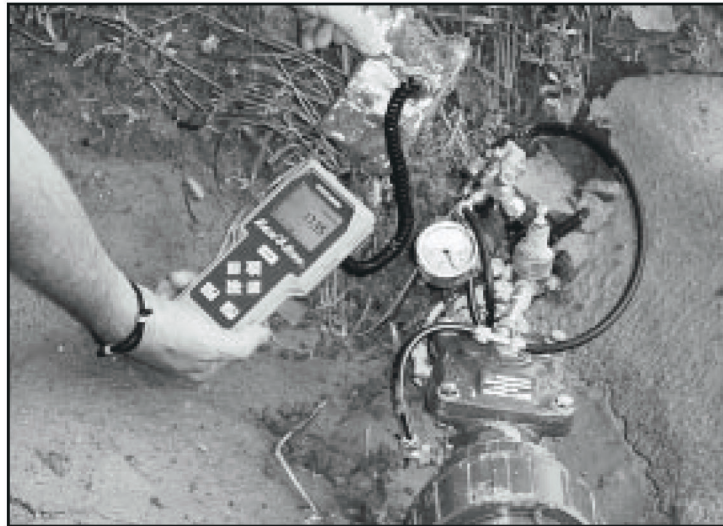
This control module was buried for 2 weeks due to flooding. Infra-red communication with the field transmitter still worked.
